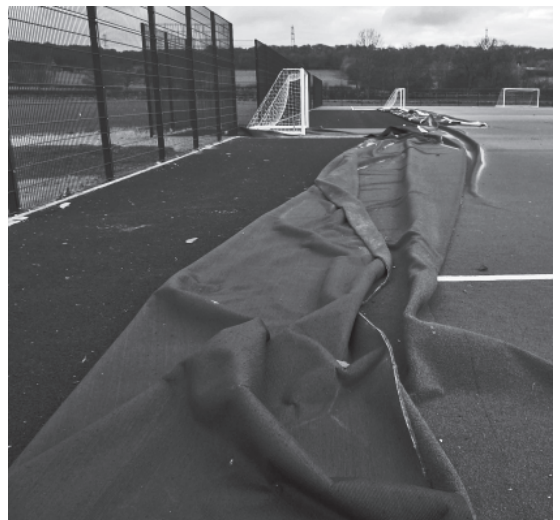
Damage caused by the high winds to the recently laid all weather pitch at St Bede's School
