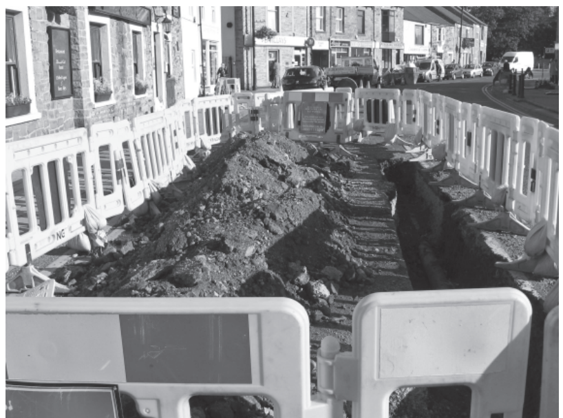
The latest hole in the road for several weeks in Front Street, courtesy of British Gas (Centrica).
