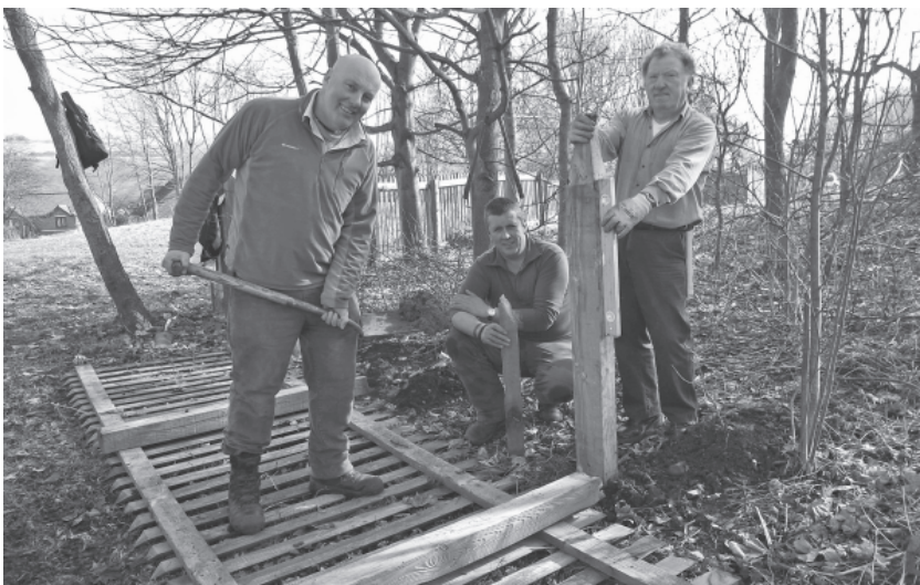
On a glorious 5th March, Mark Rothery, County Ranger for Lanchester, (left); Kevin Stock, volunteer from Sherburn (centre); and Geoff Peacock, Brook View, another volunteer, repair the fence near the Station House.
