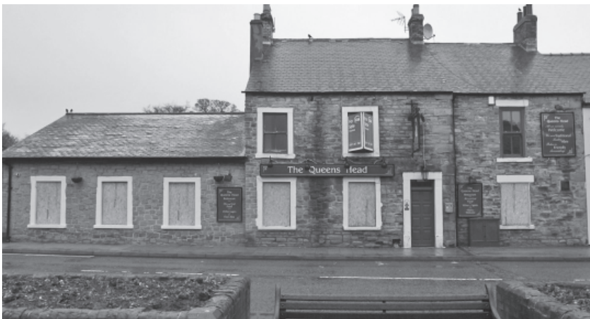
The now derelict Queen's Head where there has been a fire and floods. What is the future for this fine building?
