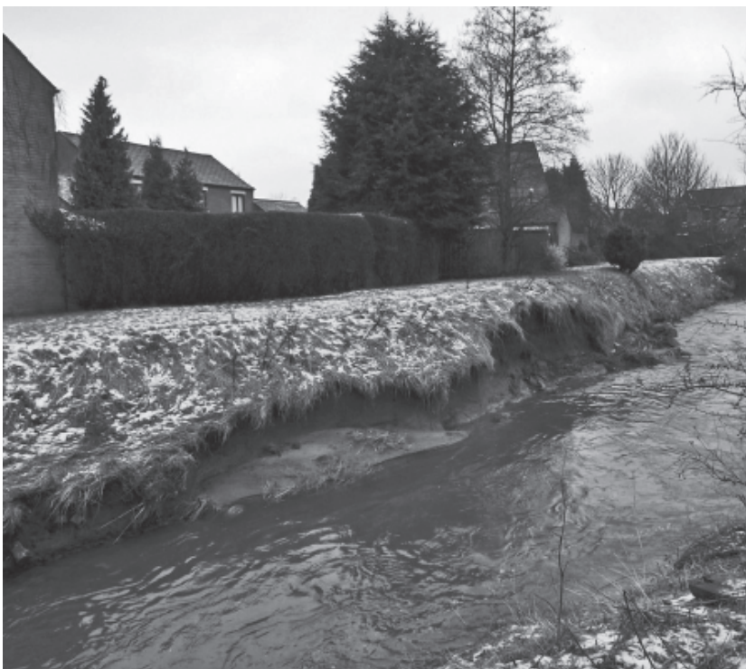
There seems to be serious erosion, due to constant flooding, on the bank of Smallhope Burn near Fenhall Park Estate.
