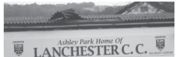
The Cricket Club does not get much luck. In a recent gale, the roof began to come off.
